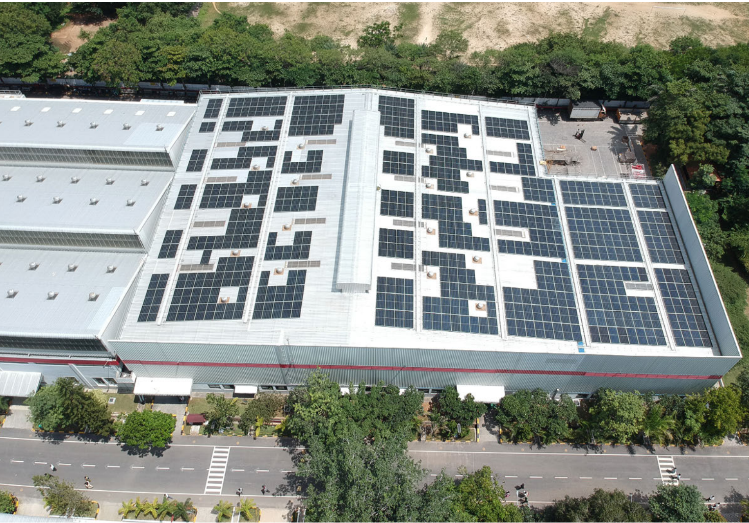
Solar panel installations at our Tamil Nadu, India, site.
