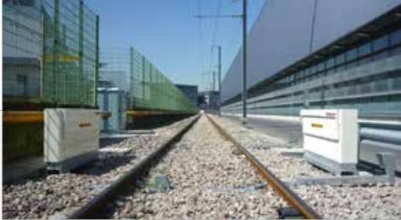
BEARING ACOUSTIC MONITOR
